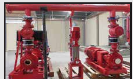
Launching of ARB Fire Pumps by Haseen Habib meeting the NFPA 20 requirements for flow and pressure-2023
