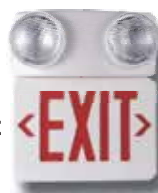
Exit Sign With Light
